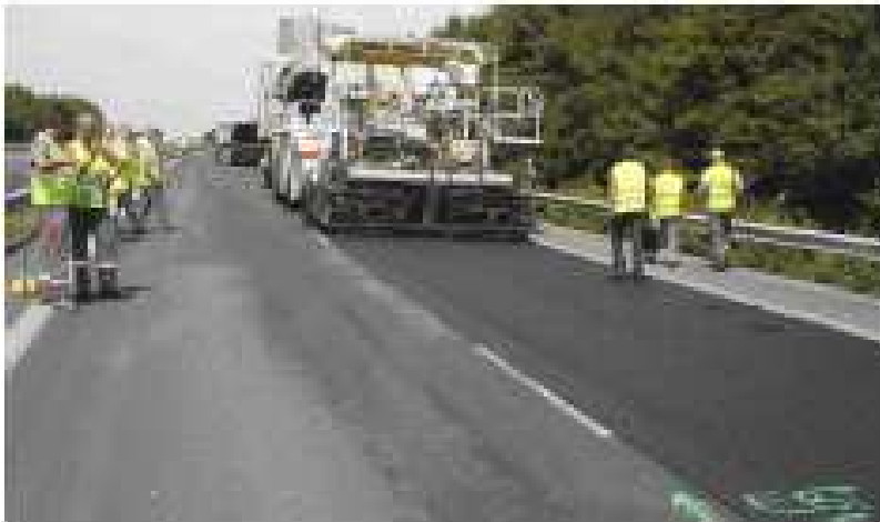
Figure 2: Paving a high-modulus LMA 2 mixture (with 50% RAP aggregate and with a new 10/20 mm grade source) at 100°C on the French A30 Highway near Amiens.
