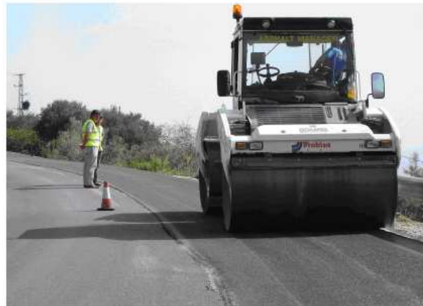
Figure 2: Compaction of in-situ recycling with emulsion with the roller (Asphalt Manager). Hereby, densities are obtained of more than 2, 2 g/cm 3
